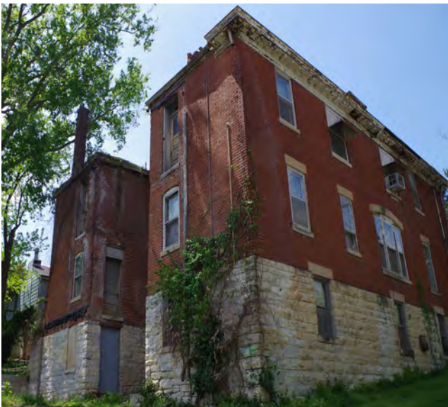
101 Jackson is vacant and has deteriorated bricks, doors, windows, and soffit.
