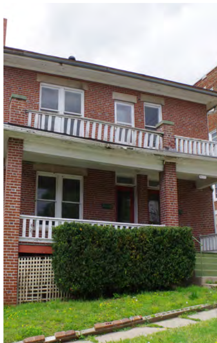
Right: The gutters and porch for 210 Lafayette are deteriorated.
