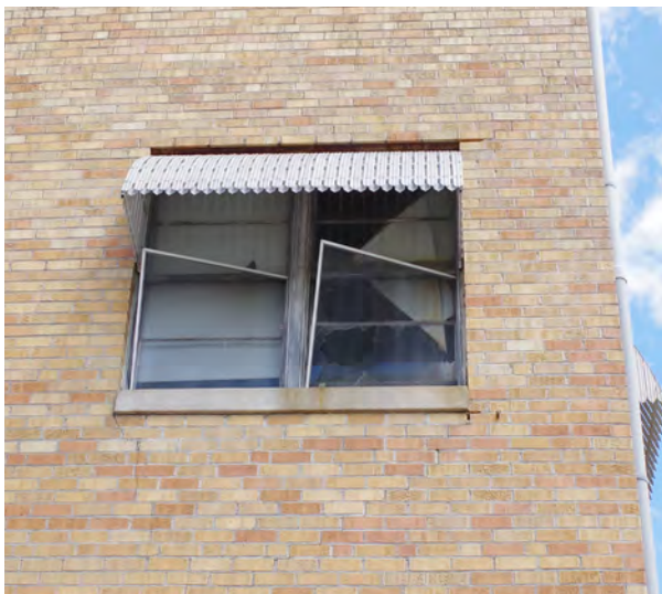
Above: Broken windows and dislodged screens at 415 Commercial Way.
