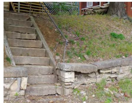
Below: The steps and retaining wall at 617 E. High are deteriorated and the retaining wall is failing.
