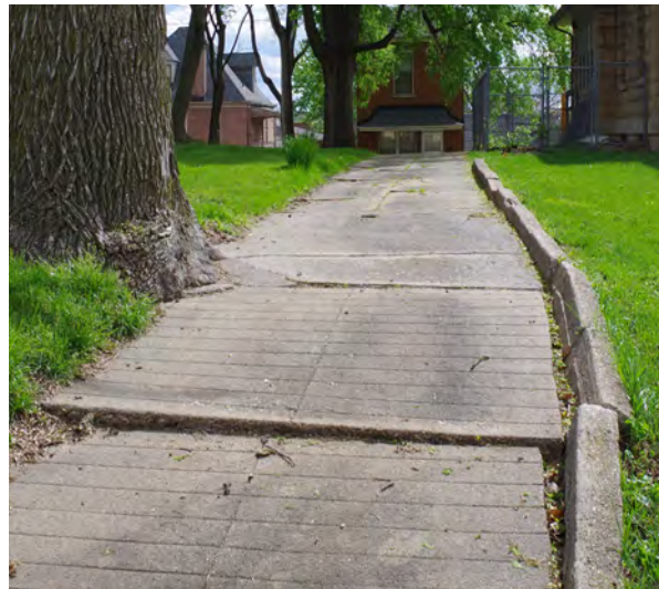
Right: The driveway for 618 E. Capitol is deteriorated.
