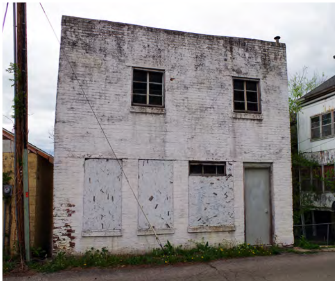
Above: 504 E. Capitol has boarded up/deteriorated windows and severe step cracking.
