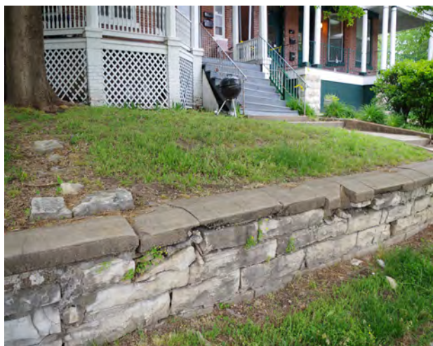
Above: The retaining wall in front of 527 E High is deteriorated.
