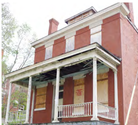
Below: The porch on the vacant, boarded-up home, 209 Jackson, is collapsing.
