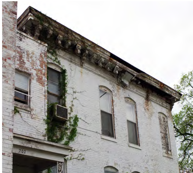
Above: 528 E. Capitol is a former single-family home that has been converted into a multi-family. The soffit, fascia, gutters, windows, and bricks on this building are deteriorated.
