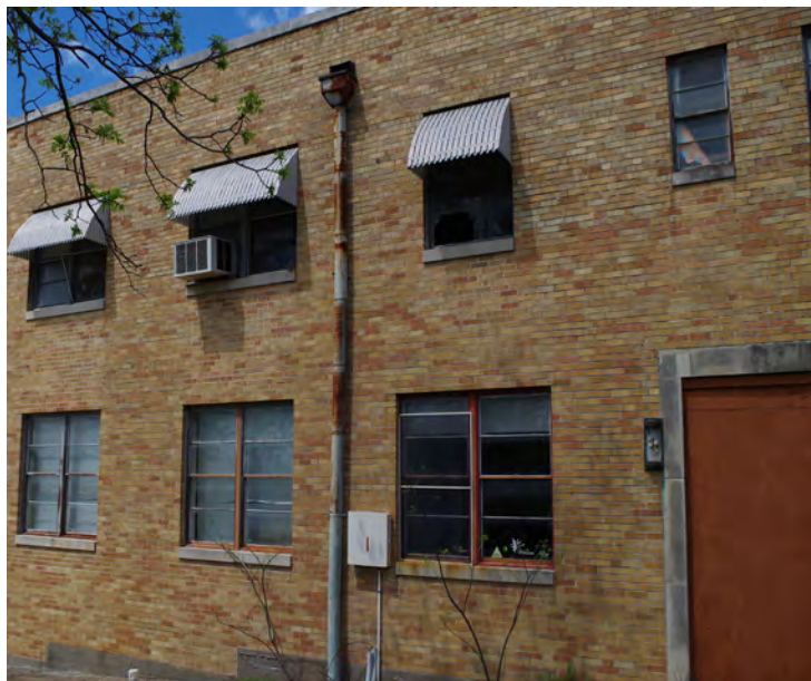
Above: 415 Commercial Way has rusted and broken windows and rusted downspouts.
