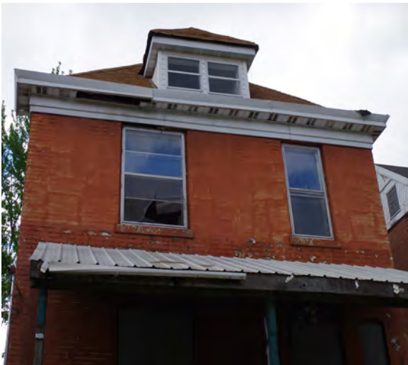
Left: 214 Lafayette is missing a section of soffit, has a deteriorated porch and is in need of tuck-pointing.
