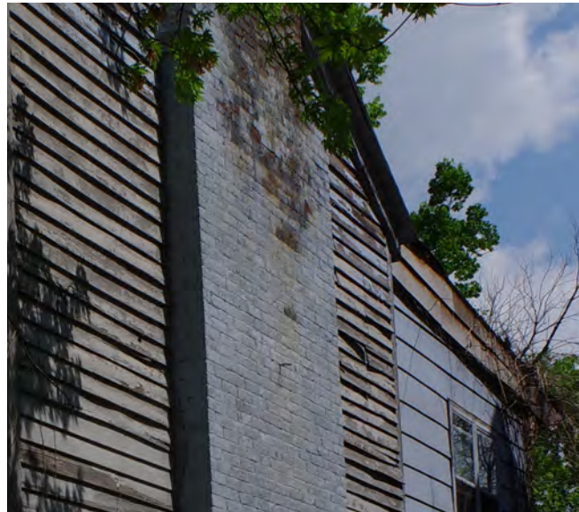
The siding on 105 Jackson is deteriorated.
