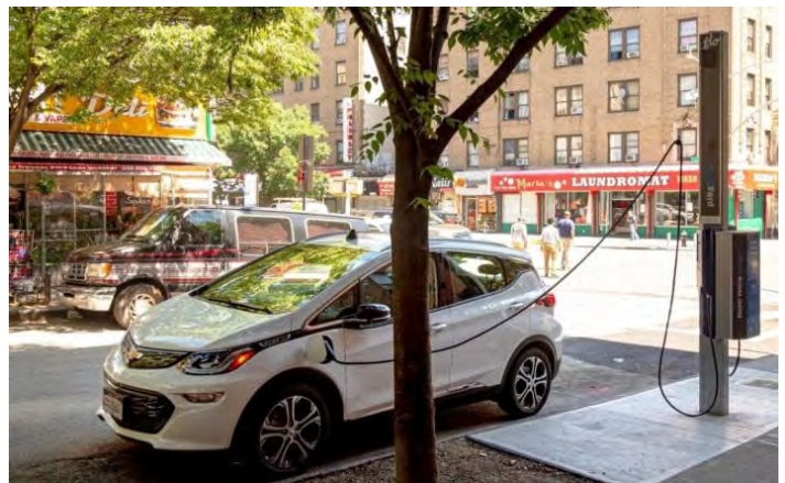
Figure 4.5: Curbside EVSE in the Bronx, New York
