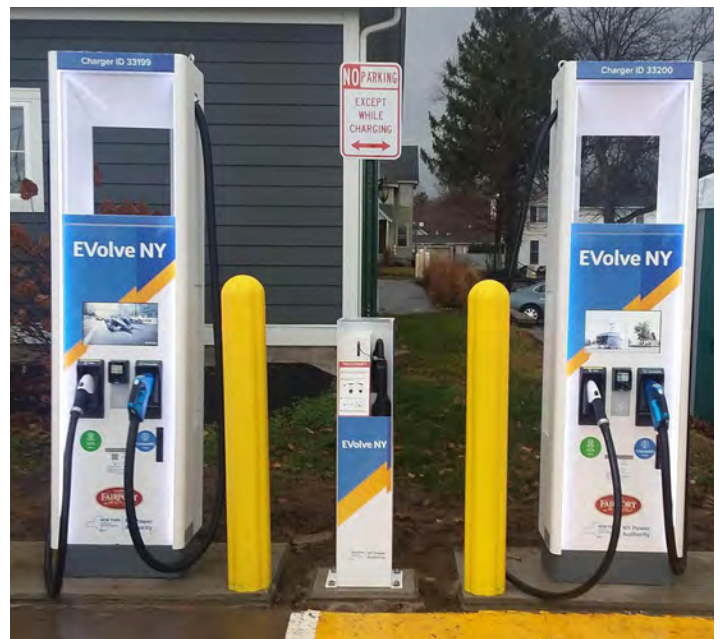
Figure 1.11: Village of Fairport Charging Stations
