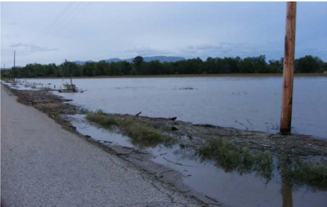
Destroyed fencing along Payette River at Idaho Blvd. – Letha, Idaho – June 2010
